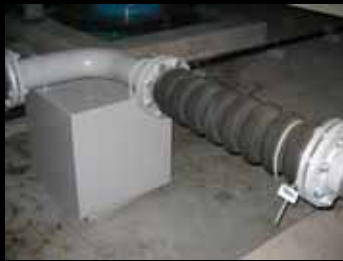
Flexible joint at service pipe
