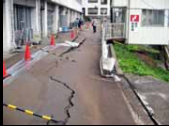
Cracks in the Road
