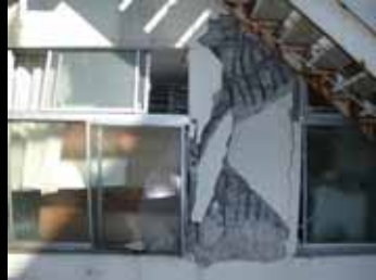
Shear fracture at RC Column
