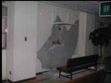
Shear cracks at RC Wall
