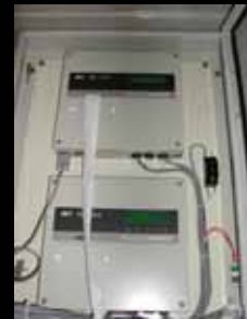
Data recorder installed at the isolation pit
